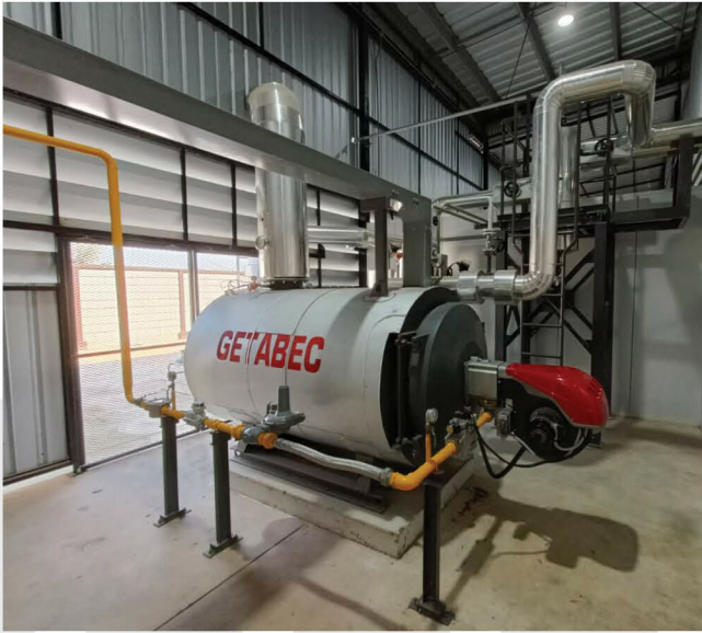
HOT OIL INSTALLATION
